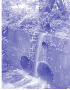
Stormwater pipes discharge directly into the environment without treatment.
